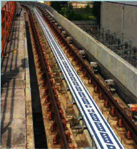
Ansaldo TramWave Third Rail Installation. Courtesy of Ansaldo STS
