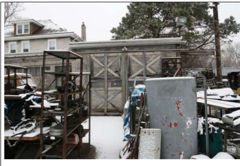
Photograph 13: Southern portion of northwest (side) elevation of the Garage/Workshop. Note the plywood construction. Looking east (January 2019).
