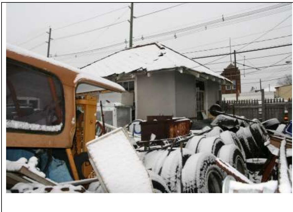
Photograph 8: Southwest (rear) and southeast (side) elevations of the Gas Station. Looking northwest (January 2019).
