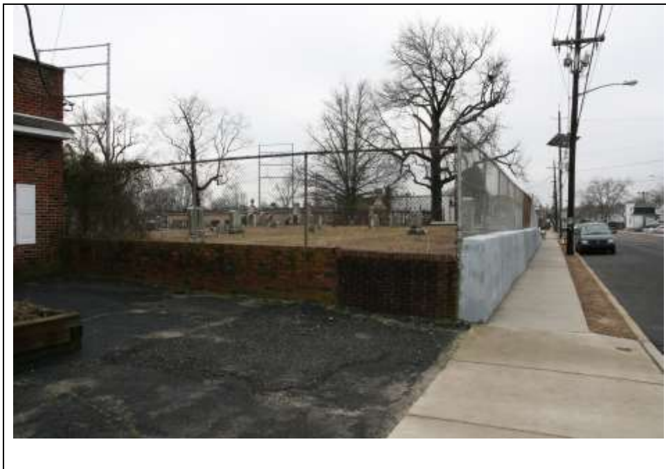
Photograph 3: Detail view of the brick retaining wall (left) and the concrete retaining wall (right). Looking southeast (January 2019).
