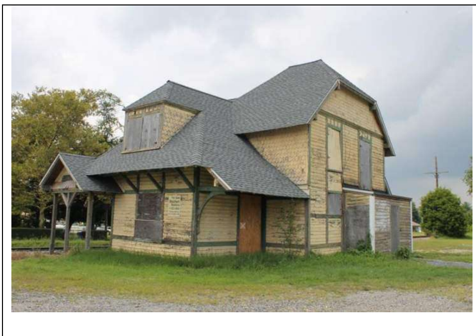
Photograph 5: Southeast (side) and northeast (rear) elevations of the Sewell Train Station, looking west (August 2013).
