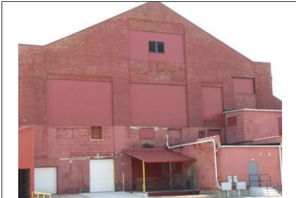
Photograph 7: Detail of northwest (rear) elevation of the 1918 furnace room (Unit A). Note the infilled window bays, which originally contained large, multi-light industrial windows. Looking south (May 2014).
