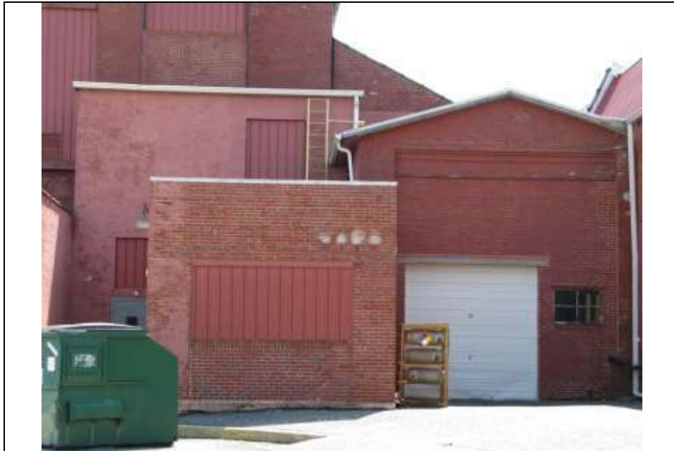
Photograph 8: Detail of small additions attached to the northwest elevation of the 1918 furnace room (Unit A). Looking southeast (May 2014).
