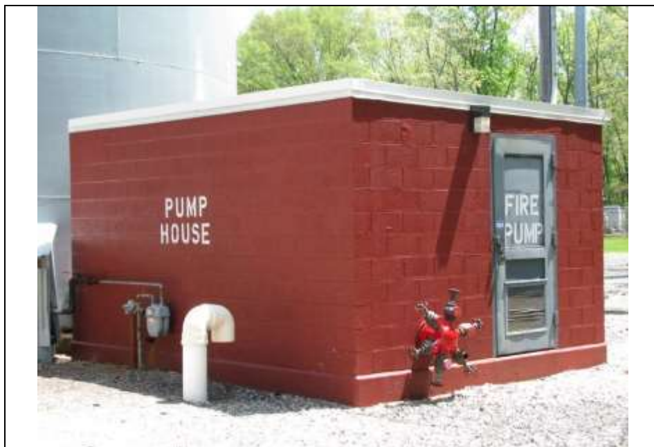
Photograph 28: Northwest (side) and southwest (front) elevations of the circa -1953 fire pump house. Looking east (May 2014).
