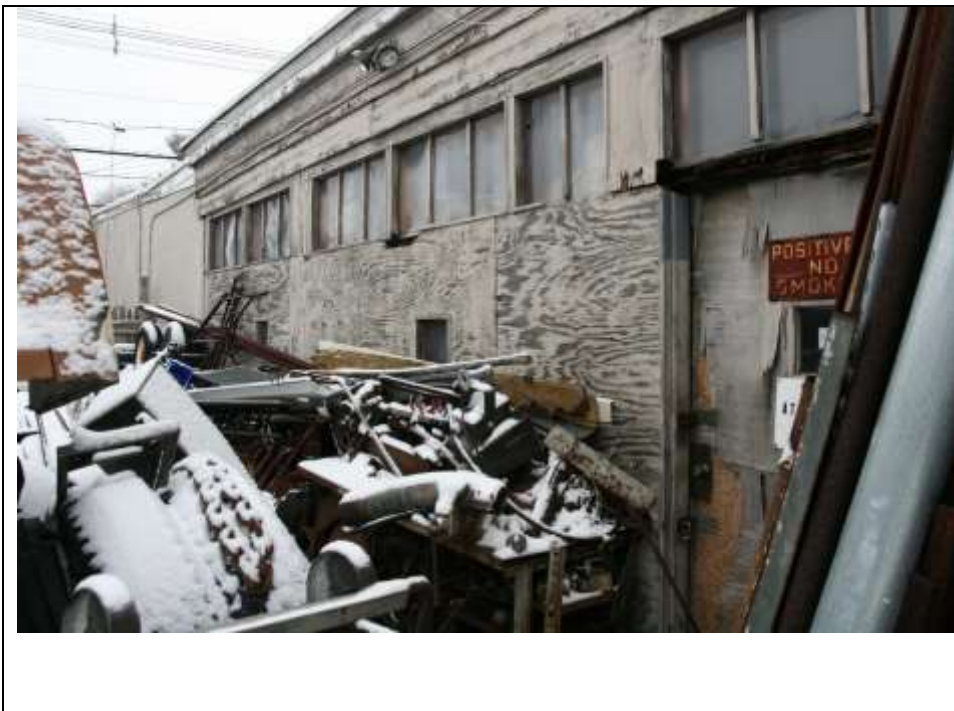
Photograph 12: Middle portion of northwest (side) elevation of the Garage/Workshop. Note the plywood construction. Looking northeast (January 2019).
