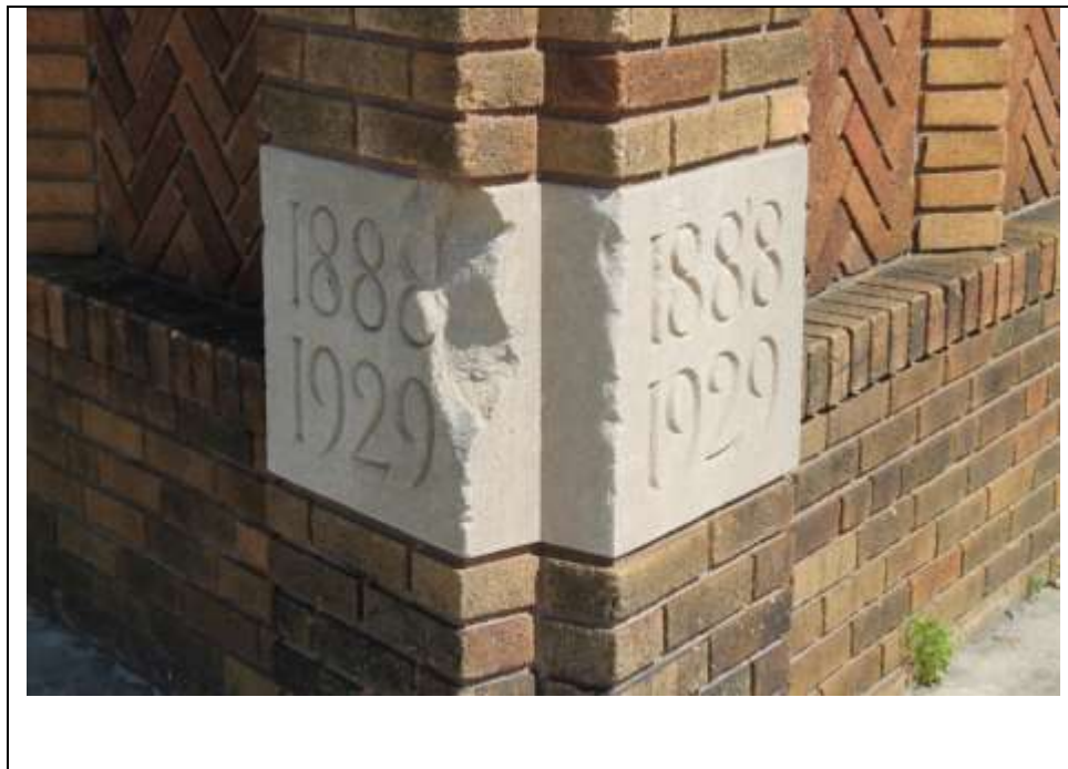
Photograph 5: Detail of the date stone at the building's southeast corner. The inscriptions 1888 and 1929 represent the year the J.R. Quigley Company was established and the year this building was erected, respectively. Looking north (May 2014).
