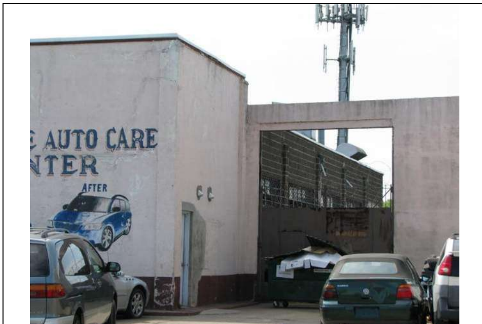
Photograph 7: West (side) elevation of Victory Garage, prior to repainting. Looking southeast (May 2014).
