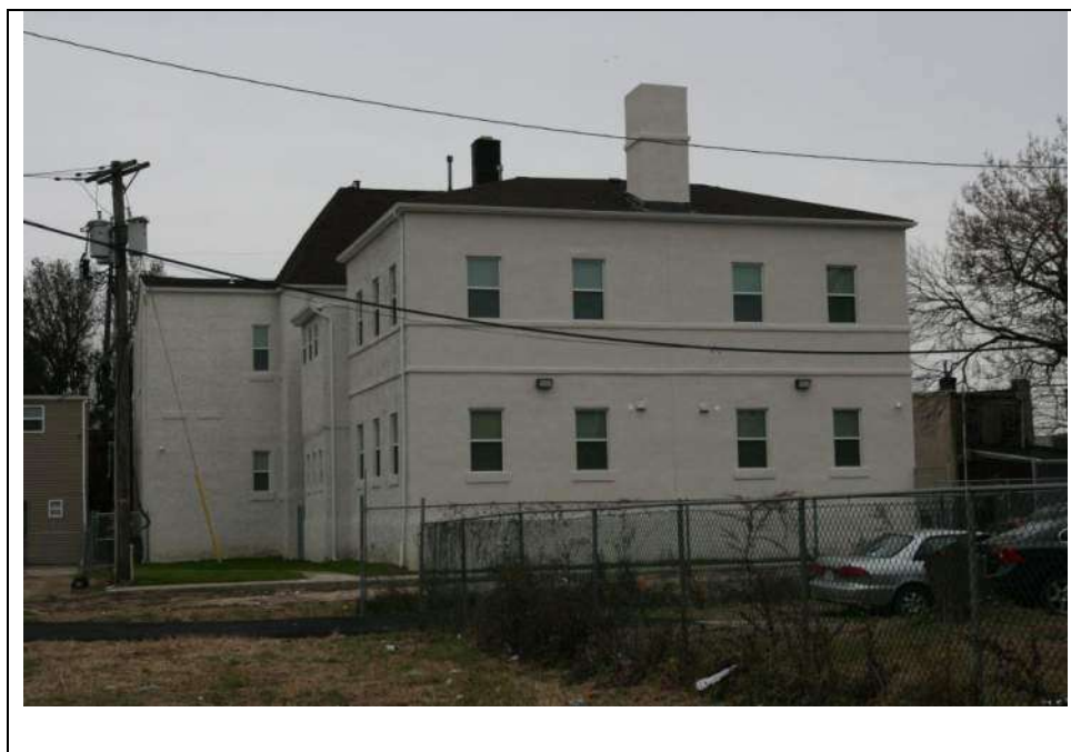
Photograph 6: North (rear) elevation of the 1888 to 1889 east wing and the circa -1900 addition. Looking southwest (December 2018).
