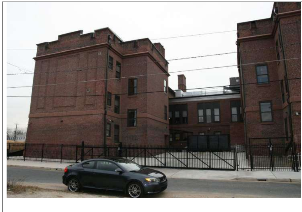
Photograph 9: South and east elevations of the western 1922 rear wing, south elevation of the original 1910-11 main building, and partial south elevation of the eastern 1922 rear wing. Looking northwest (December 2018).
