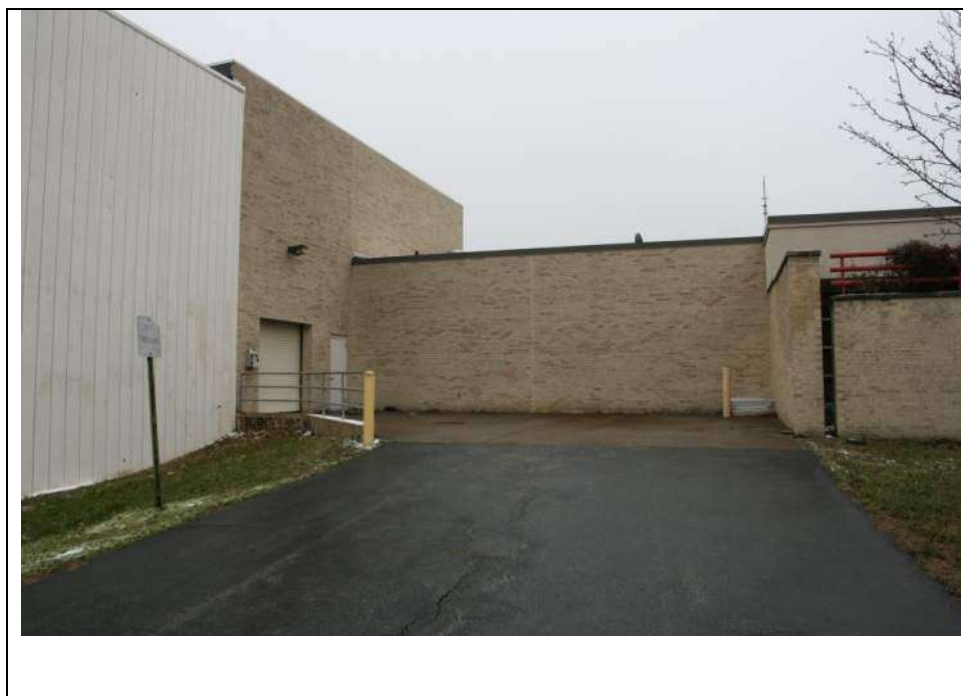
Photograph 19: Northeast (side) elevation of Block D on the right, note Block E's northeast (side) elevation and Block A's southeast (front) elevation are also visible to the left and right respectively. Looking northwest (January 2019).
