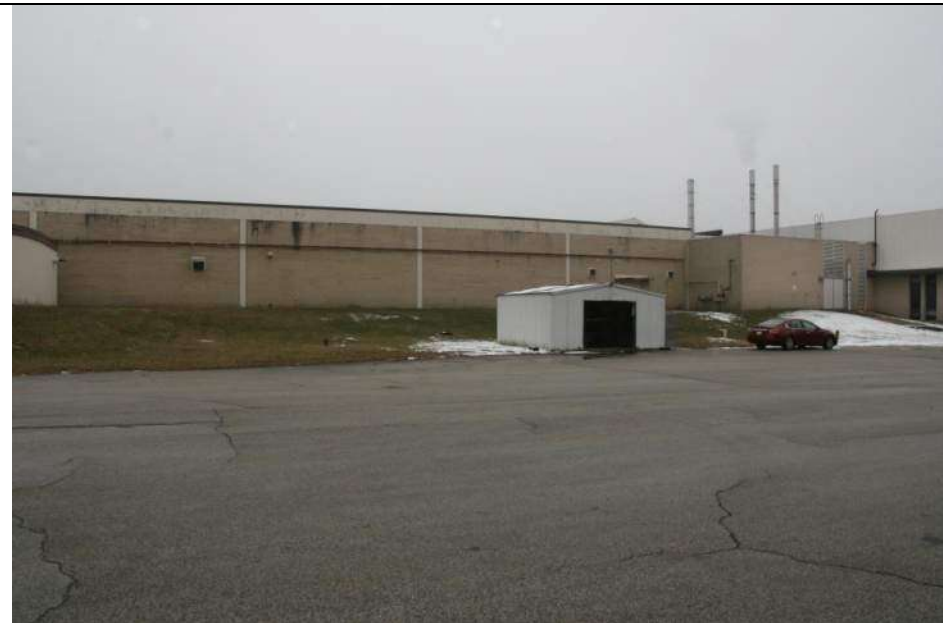
Photograph 17: Southwest elevation of Block C on the left, D on the far right, and outbuilding I. Looking southeast (January 2019).
