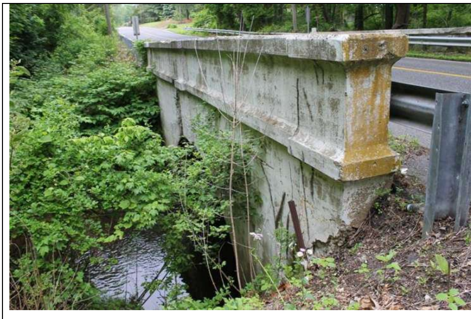
Photograph 6: South (upstream) elevation and parapet prior to the rehabilitation. Looking northwest (May 2014).
