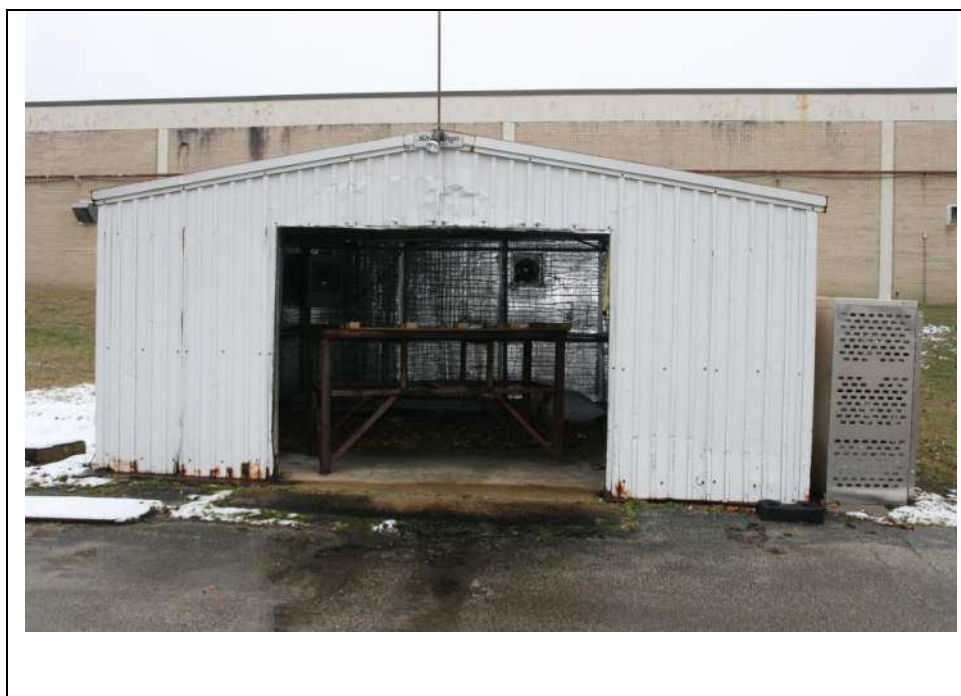
Photograph 23: Southwest elevation close up of outbuilding I. Block C is visible in the background. Looking northeast (January 2019).
