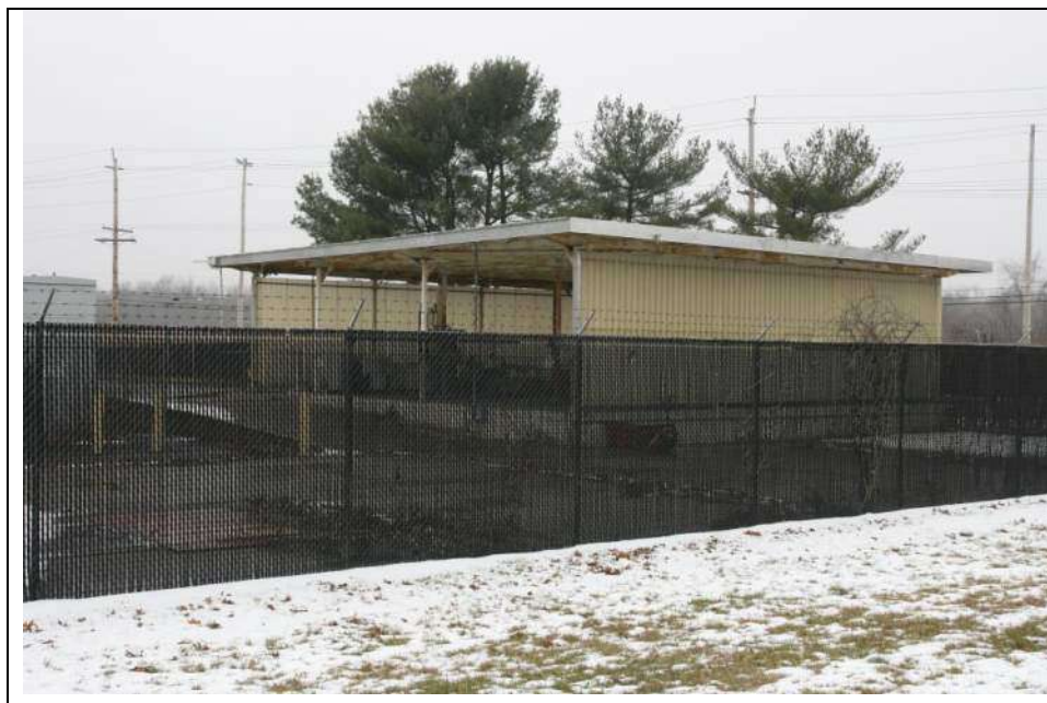
Photograph 22: Southeast (façade) and northeast elevation (side) of outbuilding H. Looking northwest (January 2019).
