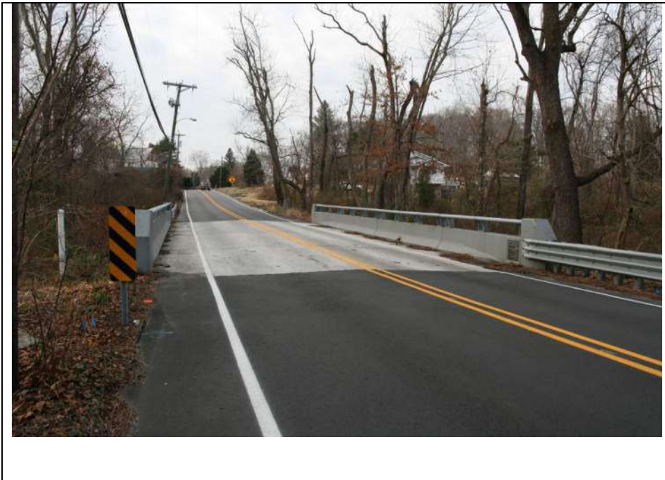
Photograph 2: Overview of the bridge, looking northwest from the east end. Note the concrete parapets with integral metal guiderails (December 2018).
