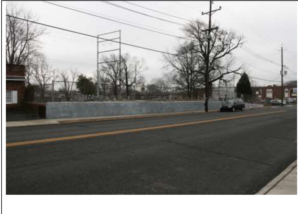
Photograph 2: View of the Presbyterian Church at Woodbury Cemetery at 400 N Broad Street. Note the concrete retaining wall. Looking east (February 2019).
