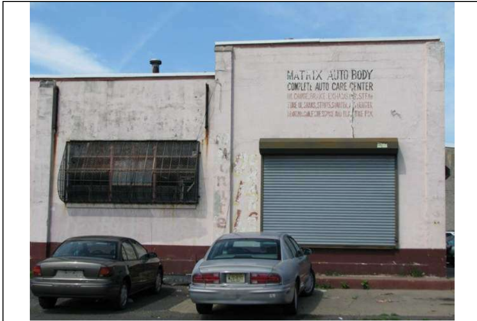
Photograph 6: Detail of east (side) elevation of Victory Garage, showing bays five and six, prior to repainting. Looking west (May 2014).
