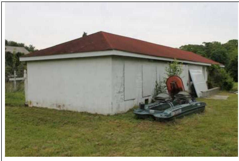
Photograph 6: Northwest (side) and southwest (front) elevations of the animal shelter at 856 Main Street. Looking east (May 2014).
