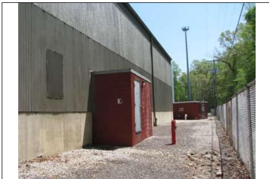
Photograph 21: Partial view of the southwest elevation of the circa -1953 Unit K. The circa -1953 fire pump house is visible in the background. Looking southeast (May 2014).
