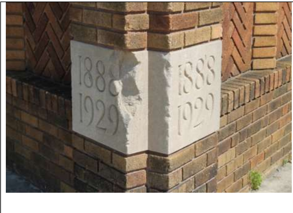
Photograph 5: Detail of the date stone at the building's southeast corner. The inscriptions 1888 and 1929 represent the year the J.R. Quigley Company was established and the year this building was erected, respectively. Looking north (May 2014).
