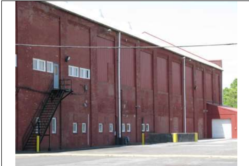
Photograph 6: Detail of northeast (side) elevation of the 1918 furnace room (Unit A). Note the infilled window bays, which originally contained large, multi-light industrial windows, and the modern windows and doors. Looking west (May 2014).
