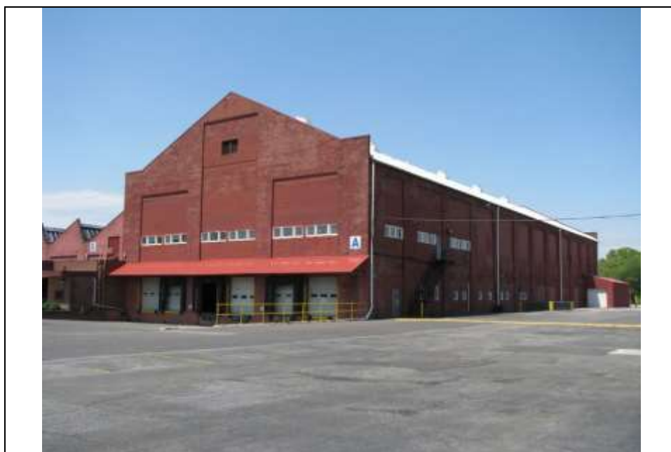
Photograph 5: Southeast (front) and northeast (side) elevations of the 1918 furnace room (Unit A). Note the metal vents that were removed ca. 2017. Looking west (May 2014).
