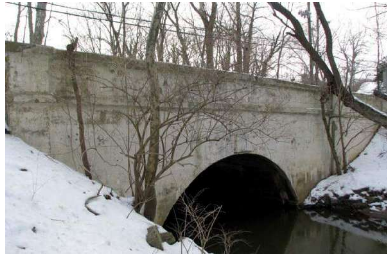
Photograph 68: Tylers Mill Road Bridge over Chestnut Branch (Structure No. 0805102), Mantua Township. View showing the south elevation. The 1926 bridge was previously surveyed and determined not eligible in 1995.
