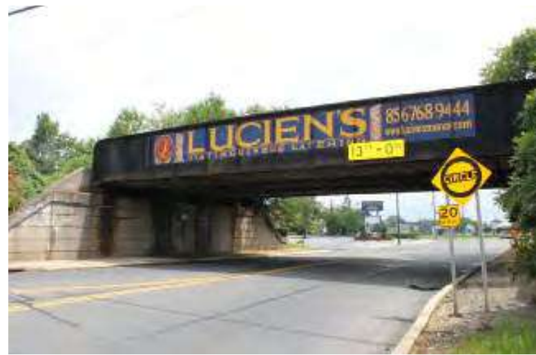
Photograph 22: West Jersey & Seashore Railroad/Pennsylvania Reading Seashore Lines, bridge over US 130, Brooklawn Borough.
