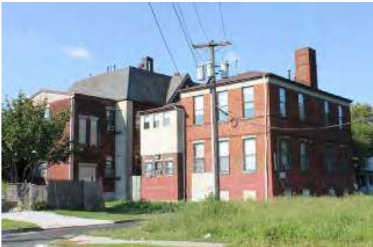
Photograph 7: Jesse Starr School (NR eligible), 823 Pine Street, Camden City. View of north (rear) and east (side) elevations, showing alterations.
